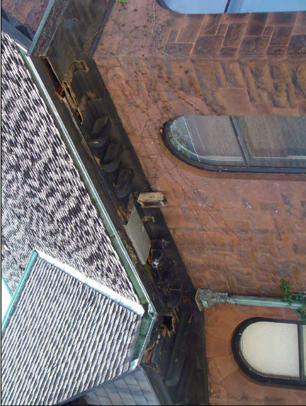
Figure 11: The Dunn Mansion- Modillion and Gutter Detail and Evidence of Damage- East Elevation, 2010, Source: CPED Files
