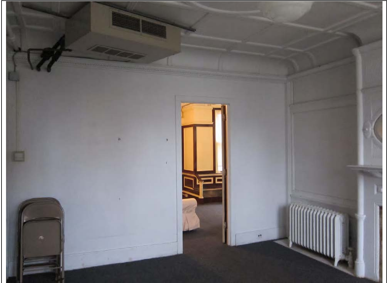
Figure 23. Nonhistoric partition wall and doorway inside parlor, facing southwest, November 2010, source: CPED files
