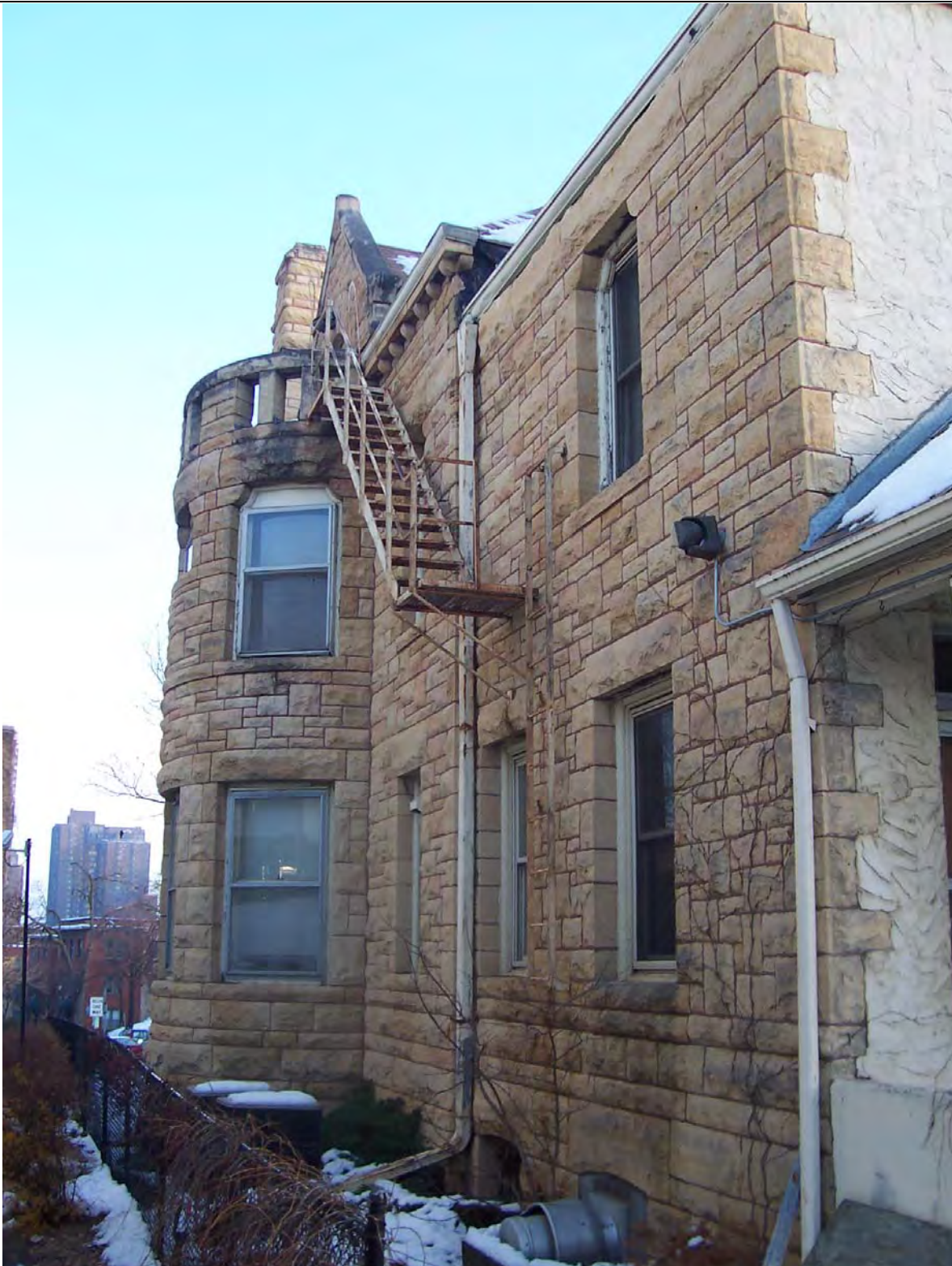
Figure 11. 131 Oak Grove, west elevation, November 2010, source: CPED files, note non-original mechanical equipment, especially at basement level
