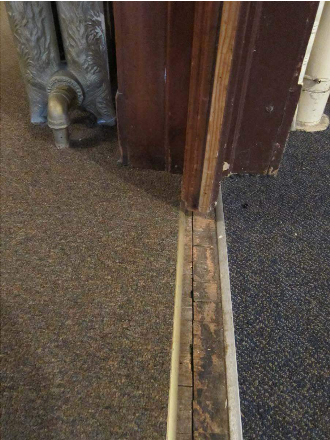
Figure 22. Original hardwood floors (likely) beneath carpeting, at pocket door where study meets dining room, November 2010, source: CPED files
