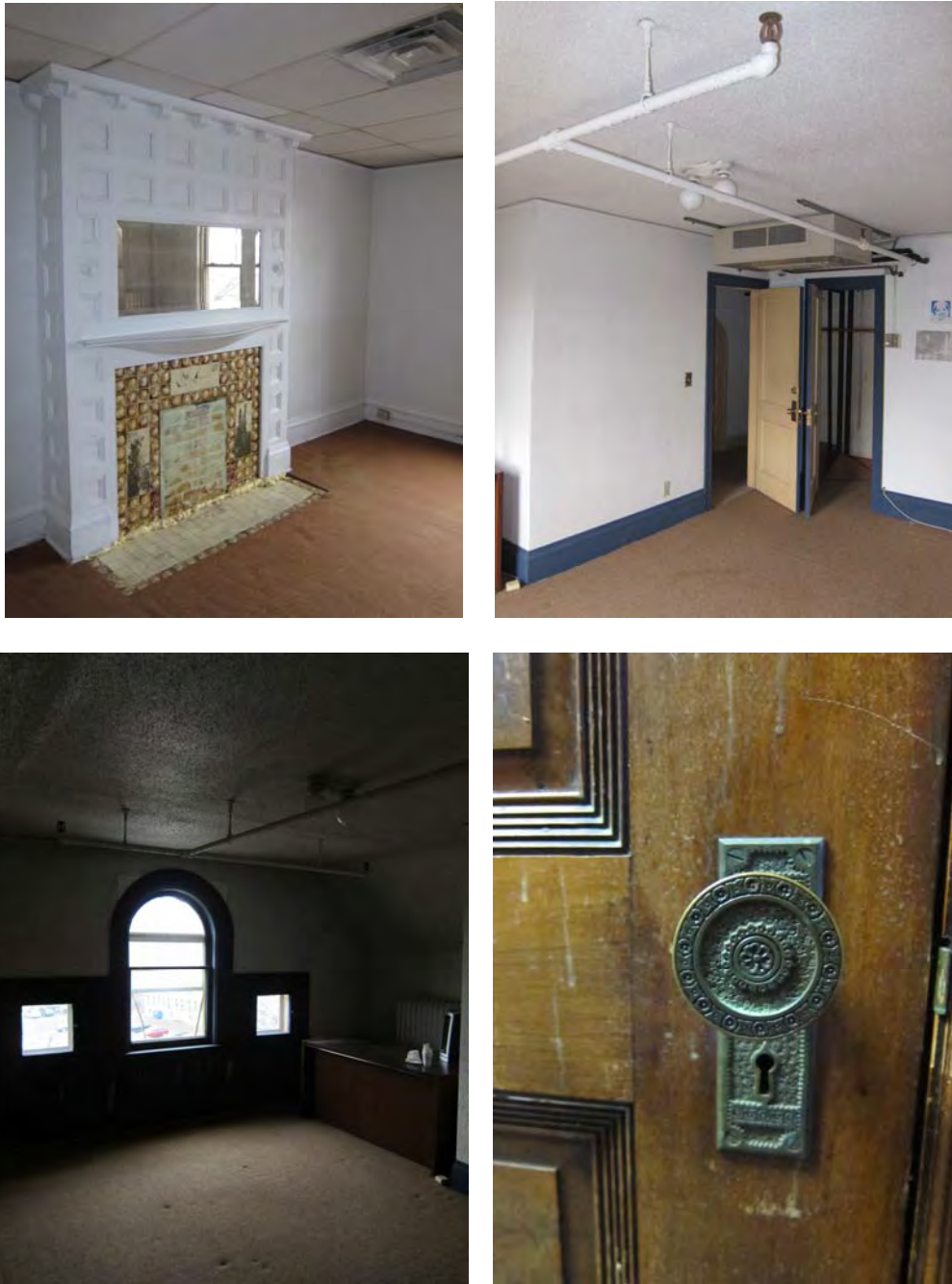
Figure 39. 131 Oak Grove, representative second and third floor secondary spaces, depicting select historic and nonhistoric materials and features, November 2010, source: CPED files
