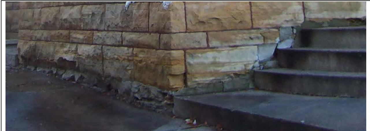
Figure 3. Masonry weathering and repairs, northeast corner, November 2010, source: CPED files
