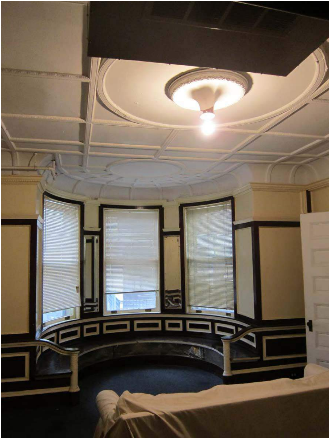
Figure 20. Bench seat and bow window in parlor, facing west, November 2010, source: CPED files, Note historic coffined ceiling with replacement light fixture and air conditioning unit
